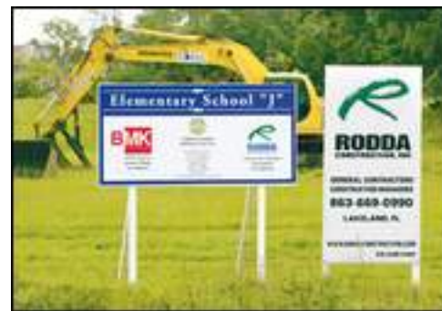
A bulldozer sits on the future site of Elementary School "J" to be built off Lakeland Highlands Road in south Lakeland. PIERRE DuCHARME/The Ledger
