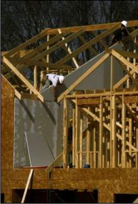
The Southside Villas are under construction in Smyrna. The Town Council is considering raising impact fees on new residential and commercial developments. STEVEN S. HARMAN / STAFF
